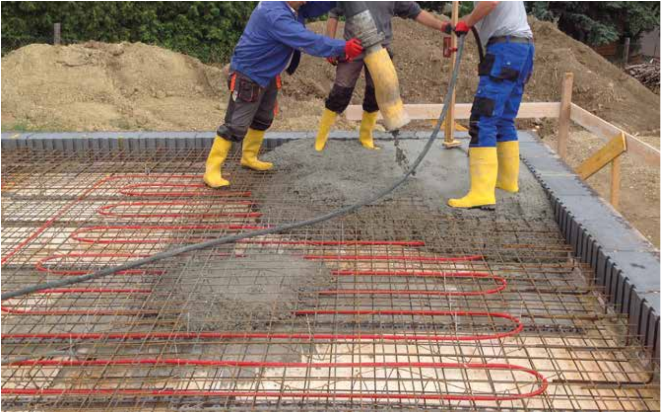
Fig. 1 | During component activation, a system of water-conducting pipelines is laid into concrete components. This is perfectly easy to accomplish. © Aichinger Hoch- u. Tiefbau GmbH
