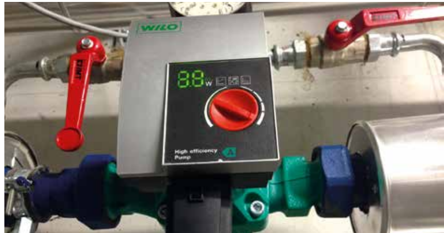
Fig. 27 | Pipe diameter, pipe length and thereby flow resistance are criteria for dimensioning the circulation pump. © FIN – Future Is Now, Kuster Energielösungen GmbH
