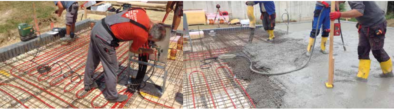
Application examples of thermal component activation: Assembly of pipelines, pressure test and placing of concrete for the ceiling. © Aichinger Hoch- u. Tiefbau GmbH
