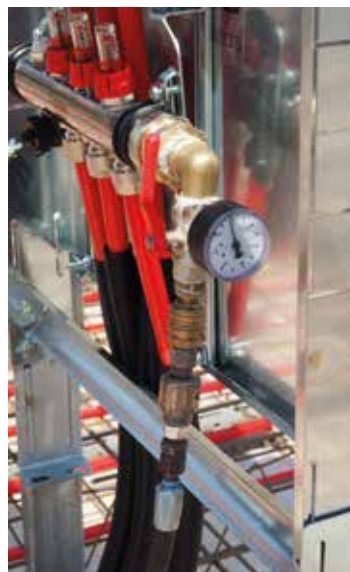
Fig. 44 | bottom left and right The pressure test is done before, during and after concrete work. © Thomas Schönbichler/CL; © Aichinger Hoch- u. Tiefbau GmbH
