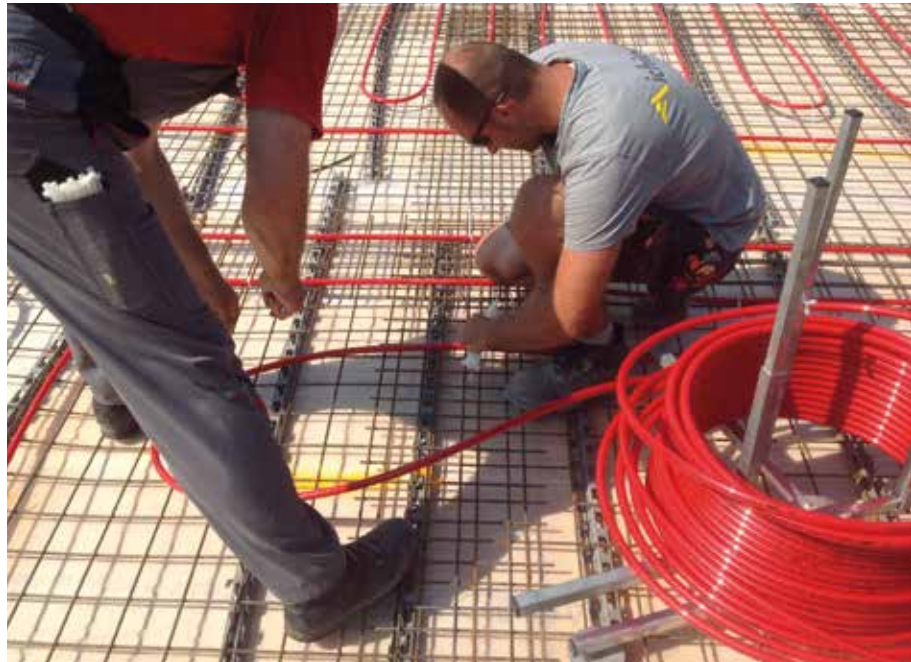
Fig. 3 | The installation of heating and cooling registers into the ceiling can be done quickly, easily and therefore economically. © Aichinger Hoch- u. Tiefbau GmbH
