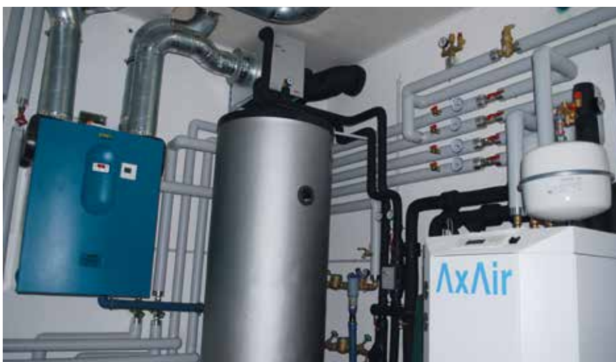
Fig. 24 | The power house with heat pump, hot water boiler, circulation pump and distribution lines, etc. is assembled manageably in the smallest possible space.
